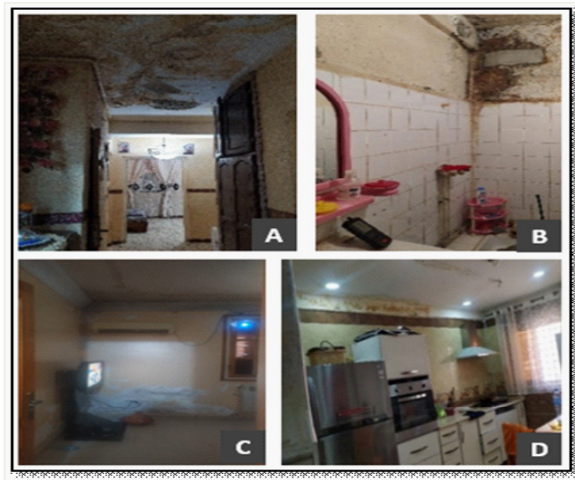
Figure 2. Damp stains observed in the apartment. (Source: Authors, 2021)
